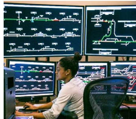
An Amtrak employee at the Szabo Control Center. This Chicago facility is one of five Amtrak dispatching offices that control 2,500 trains with nearly 900,000 daily passengers.
